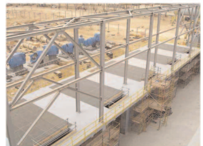
Station pompage eau de mer (Caillebotis)
